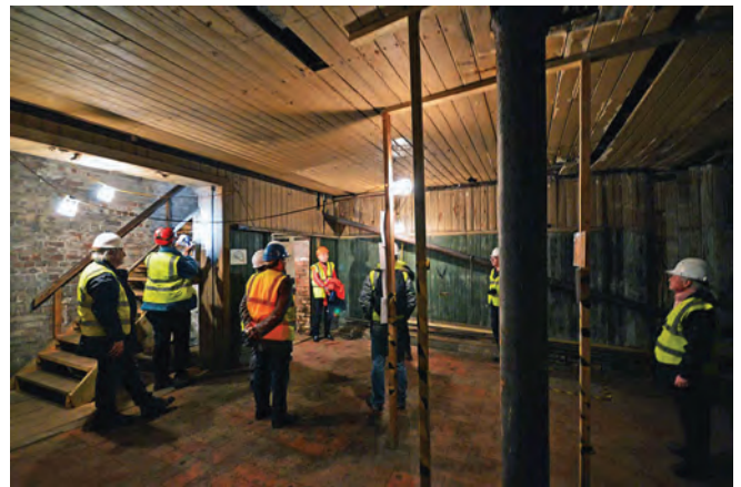
The original Rocks Railway low station waiting room, with timber panelling concealing steelwork with reinforced concrete infill
